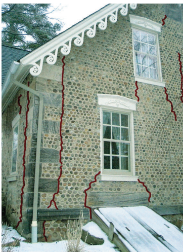
Fig. 5 (below right) Crack running from doorway lintel to sill above.
