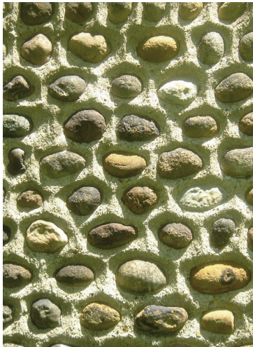
Fig. 2 (above) Projecting mortar joints create a honeycomb effect.
